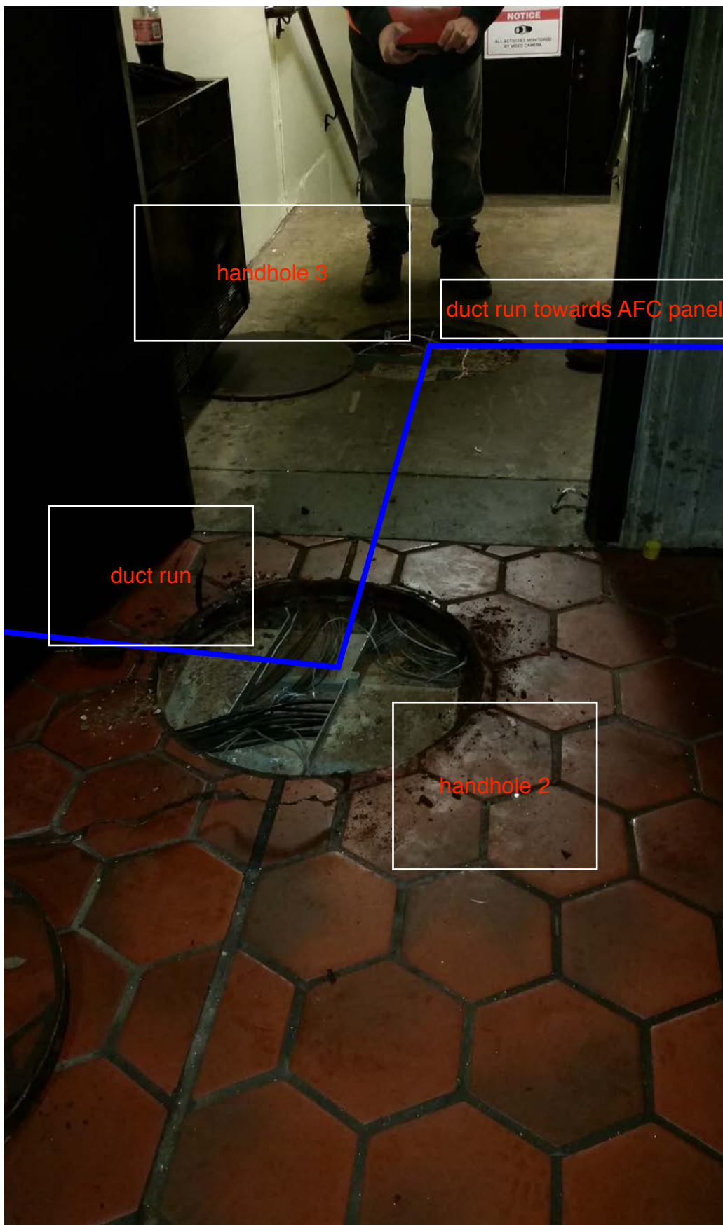
Photo #3 – E07 West Hyattsville: Duct run from handhole 2 to handhole 3
