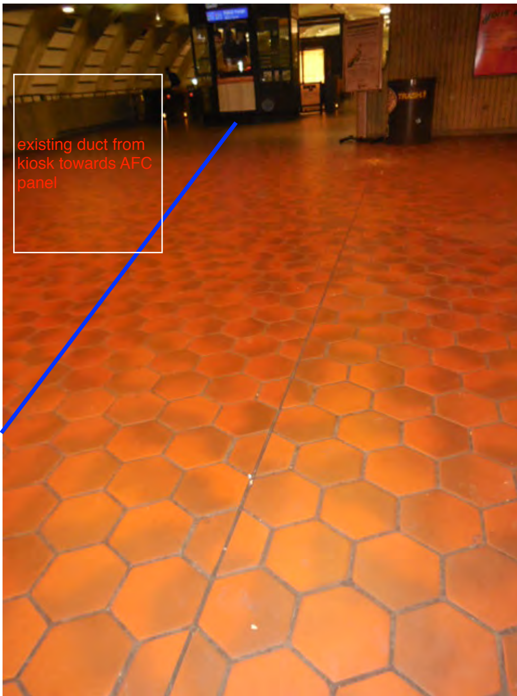
Photo #1 – E05 Georgia Avenue: Duct run from kiosk towards handhole 1
