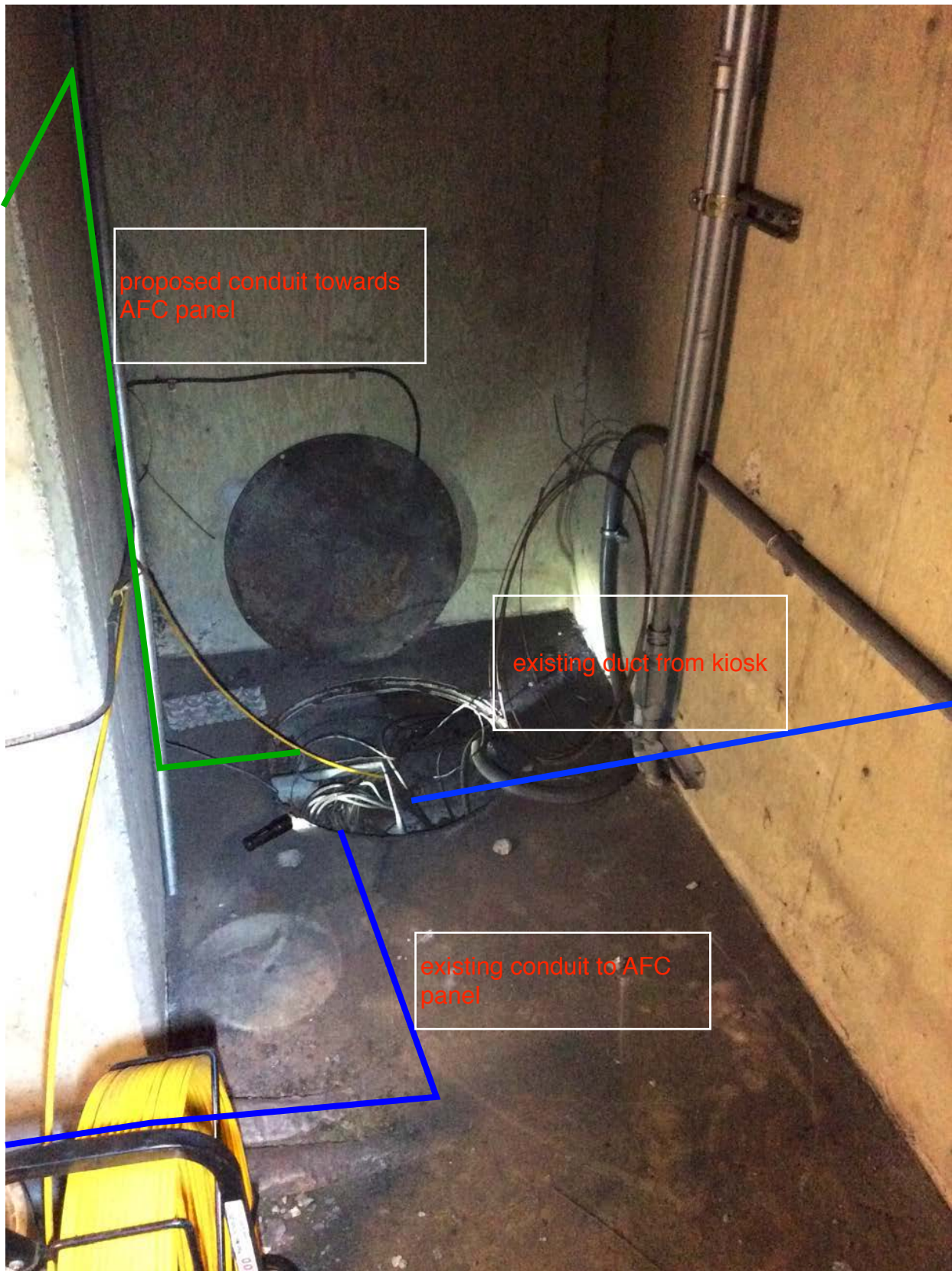
Photo #2 – E05 Georgia Avenue: Duct run into handhole 1 and conduit from handhole 1 to AFC panel
