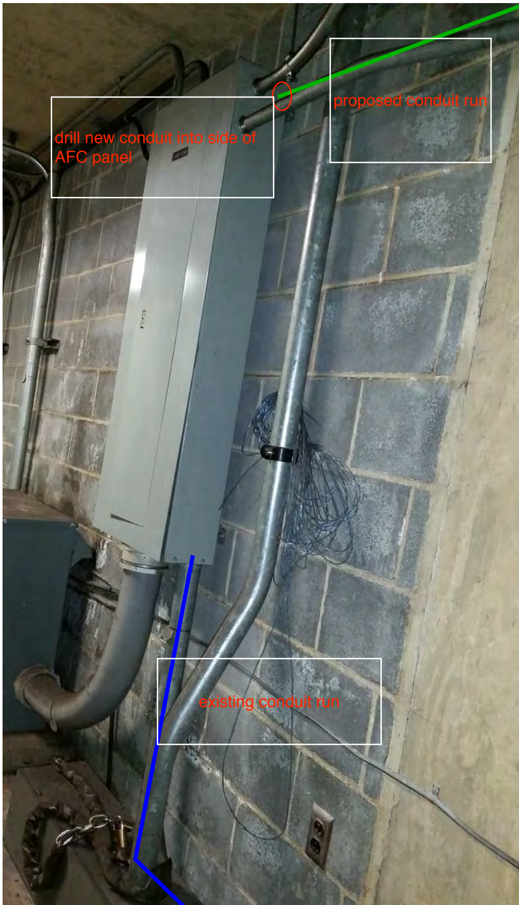
Photo #4: E05 Georgia Avenue: AFC panel with proposed conduit run from handhole 1
